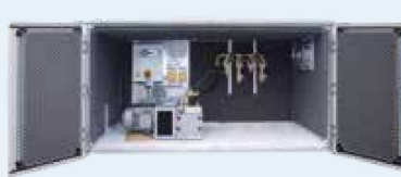
Concrete external cabinet
