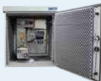
L metal external cabinet
