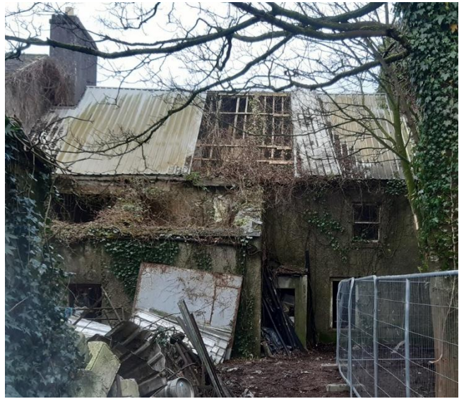
Image 11. Lean-to extension and main roof collapse
