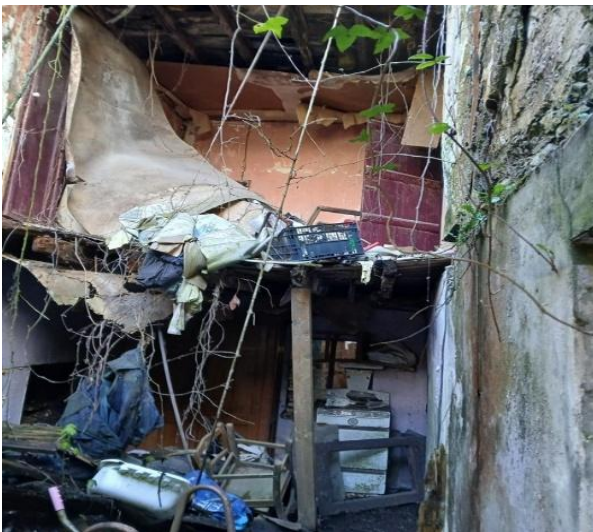
Image 12. Collapse of first floor
