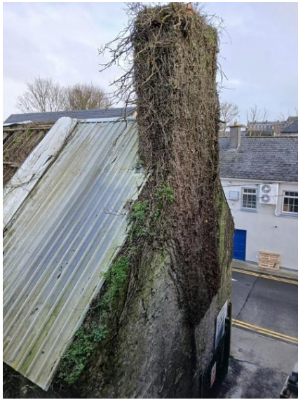
Image 10. Chimney stack leaning
