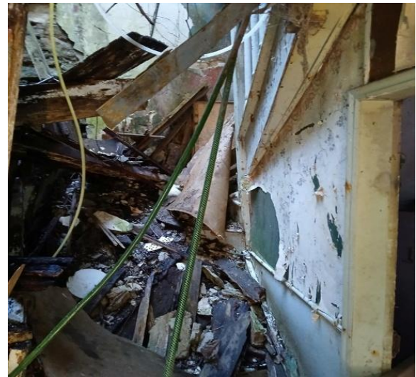
Image 13. Collapse of stairs and landing
