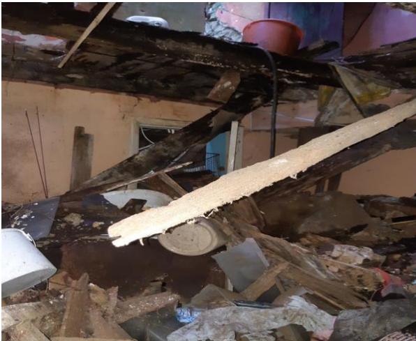
Image 14. Collapse of first floor
