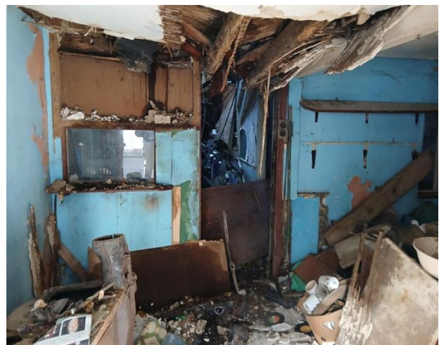
Image 15. Collapse of first floor
