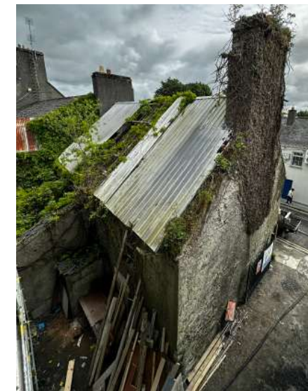
Fig.20: View of overgrowth on roof and chimney
