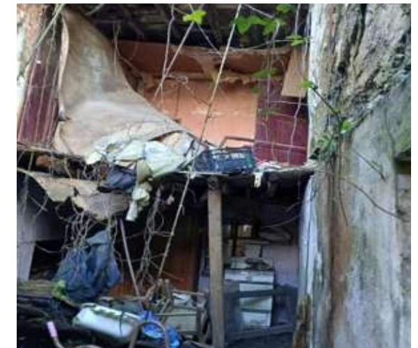
Fig.22: Interior View of Collapse
