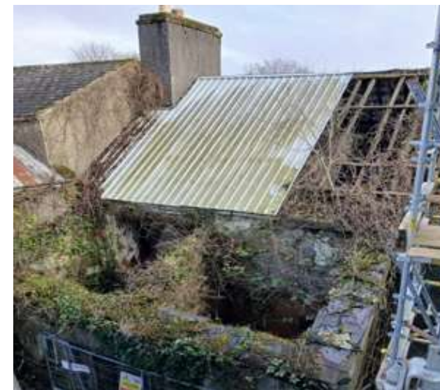
Fig.19: View of collapsed Roof
