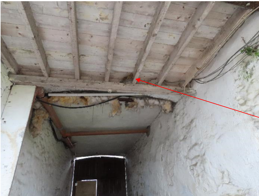
Photo 9 – access to rear of building via archway between Dooley's pub and Dunlo Hill terrace. Several swallows' nests were recorded on roof timbers
