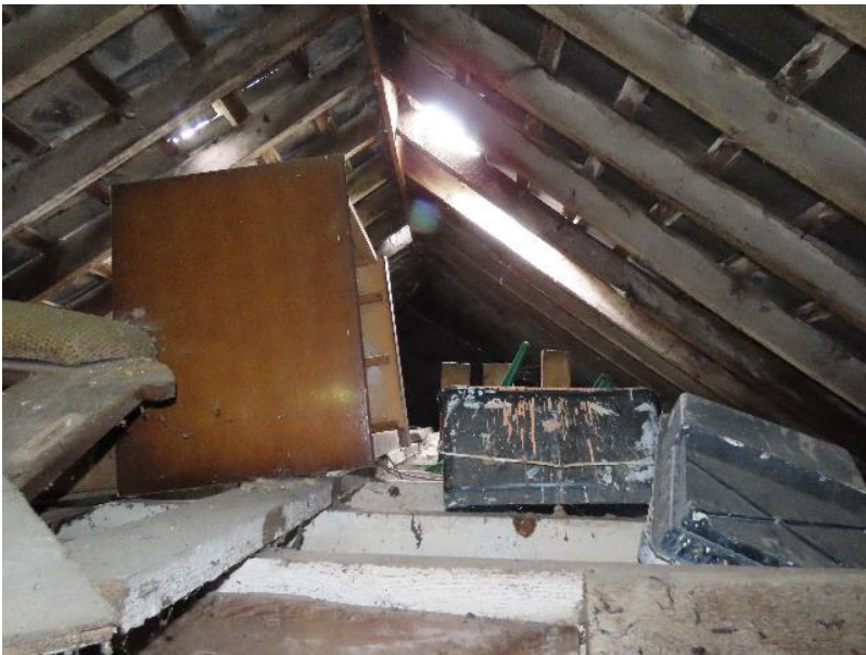
Photo 33 - Attic of Property 4 with void in roof
