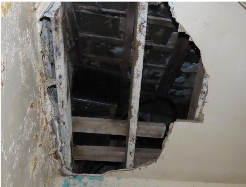
Photo 21 - Hole in upstairs ceiling of Property 1 in Dunlo Terrace
