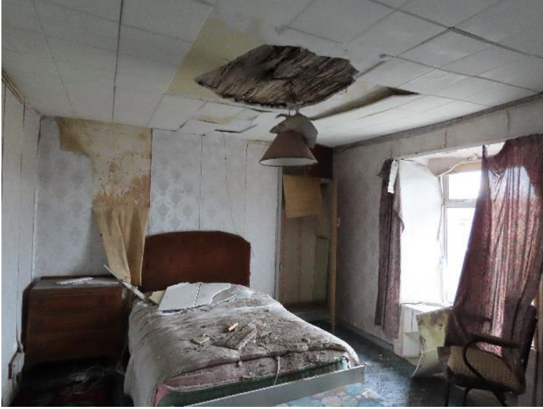
Photo 57 – bedroom with damaged ceiling
