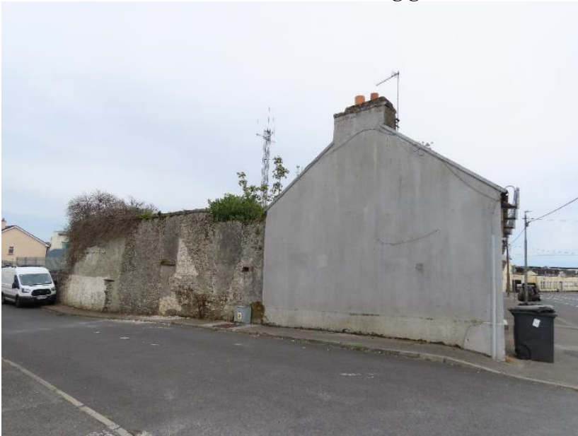
Photo 1 – western end of Dunlo Hill terrace – western gable and stone wall to rear
