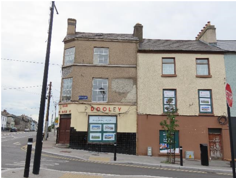
Photo 7 - Eastern elevation of Dooley's pub on corner and adjoining 3 storey property (Property No. 9)
