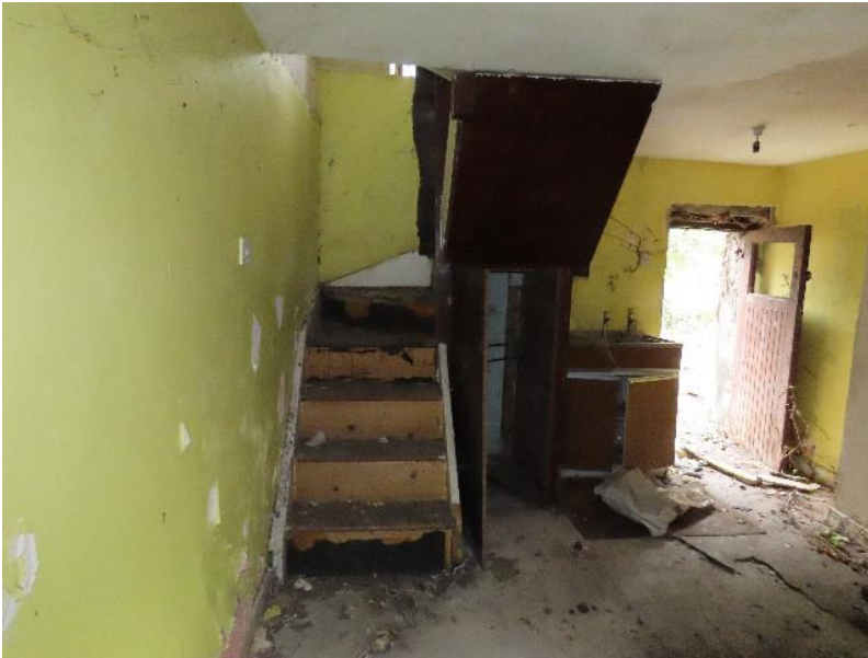
Photo 19 - Interior of Property 1 in Dunlo Hill Terrace
