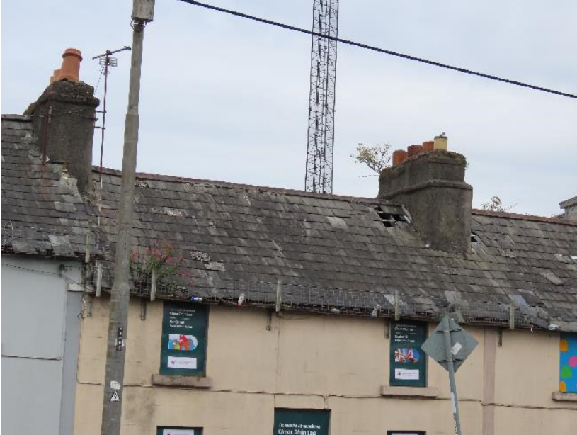
Photo 5 - Roof of Property 5 with hole around chimney stack
