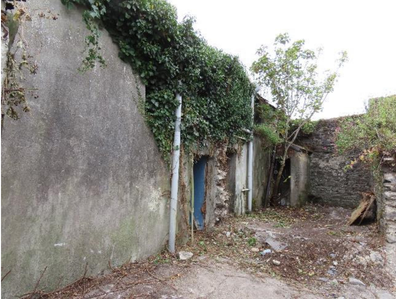
Photo 14 - Rear of Dunlo Terrace – westernmost section. Access to each unit was via the rear door
