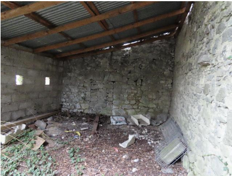
Photo 15 – Lean-to stone shed to rear of westernmost property in Dunlo Terrace. This building was considered to have potential as a bat roosting site
