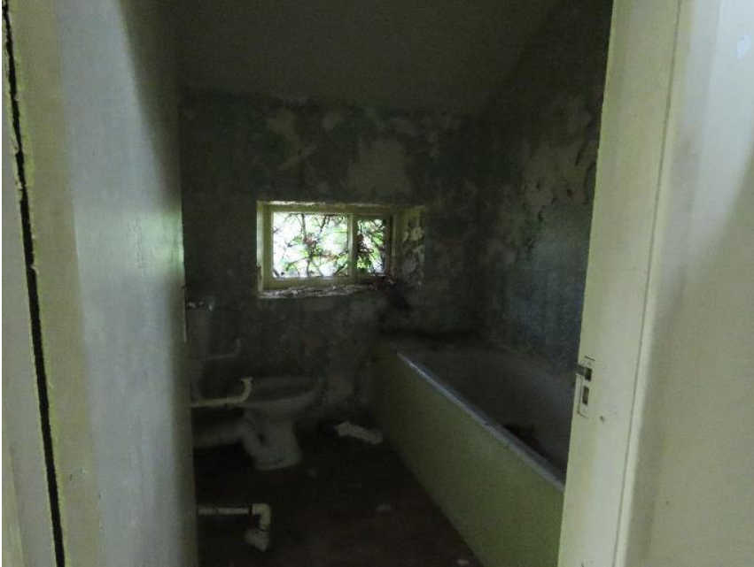
Photo 32 – upstairs bathroom in Property 4
