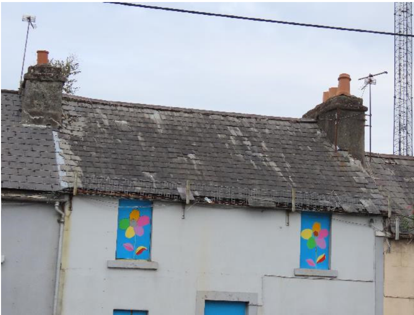
Photo 4 - Property 4 – showing poor condition of roof. Wire slate guard in place to catch falling slates
