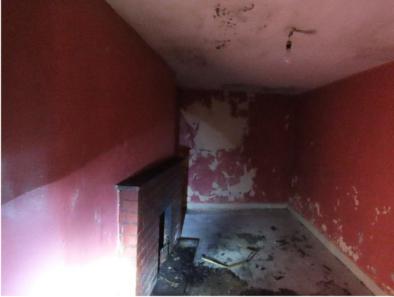
Photo 18 - Interior of Property 1 in Dunlo Hill Terrace
