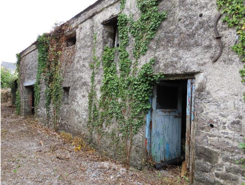
Photo 61 – stone outbuildings to rear of Property 9. These buildings were considered to have the greatest potential for roosting bats but no bats were recorded
