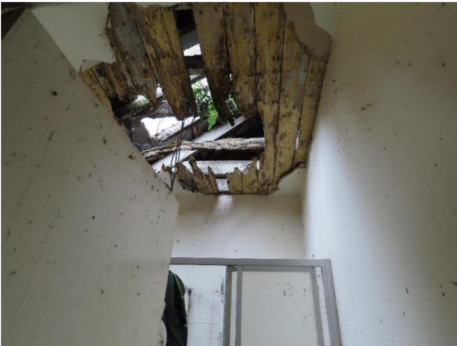
Photo 38 – damage to ceiling in Property 6
