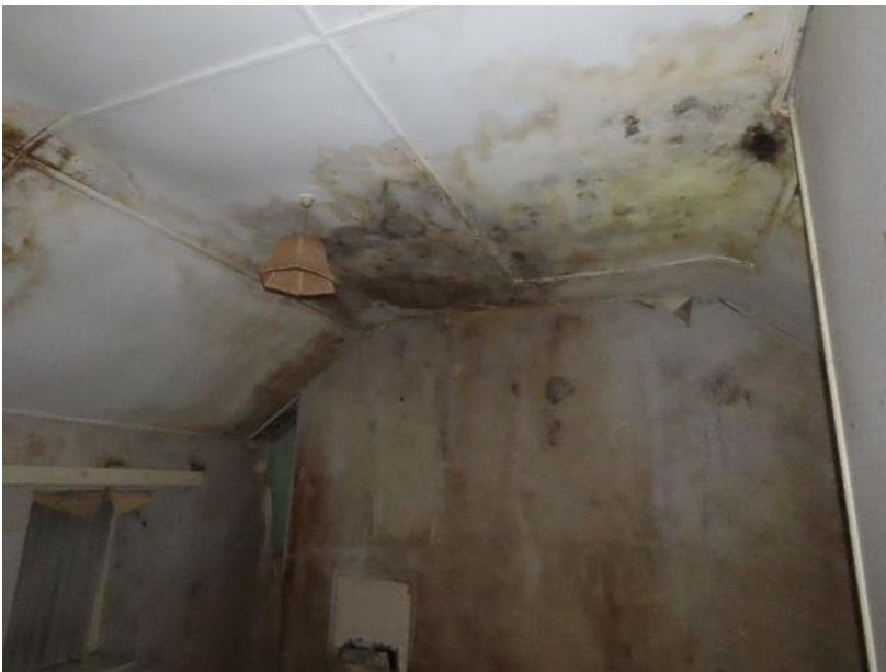
Photo 36 – damage caused by water egress in property No 6
