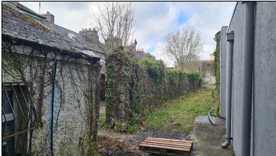
Plate 4 Facing SW from NE extent of site showing old boundary wall and gate pillar
