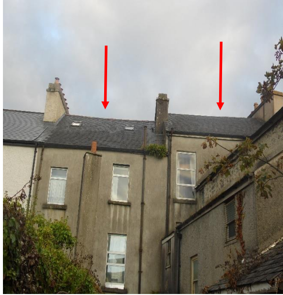
Slates to Roof of two Townhouses strongly presumed ACM's
