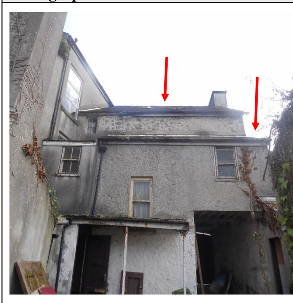
Slates to Roof of extension to rear of (Dooleys)Townhouse strongly presumed ACM's
