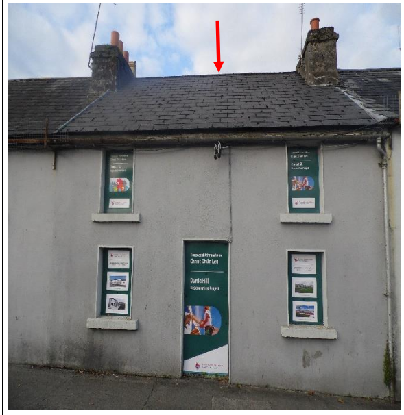
Slates to Roof of Terraced House #5 are strongly presumed ACM's
