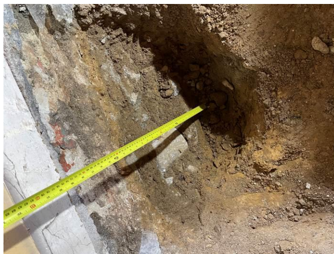
Photograph 5: Shallow depth of bearing stones under external / party walls of the existing dwellings (Unit 02)
