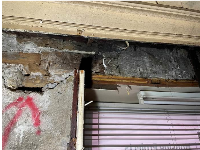
Photograph 16: Typical example of the nature and condition of the timber lintels and beams in the public house area
