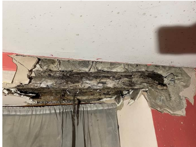
Photograph 8: Condition of Timber Lintels in Unit 01
