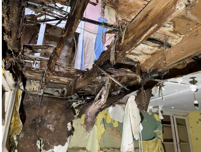
Photograph 32: First floor joists were found to be in this dilapidated condition within a number of the residential units
