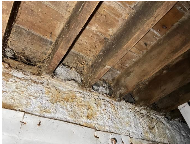
Photograph 39: Dilapidated condition of the timber floors and floor joists on the ground floor of the public house area
