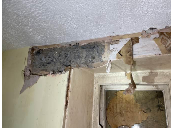
Photograph 10: Concrete & stone lintels were also noted in places within the residential properties
