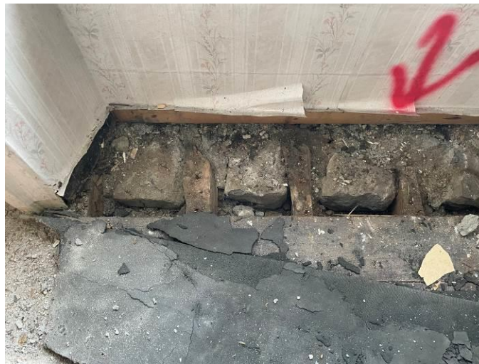
Photograph 31: Example of first floor timber joists abutting a stone wall. The joists were found to be in good condition
