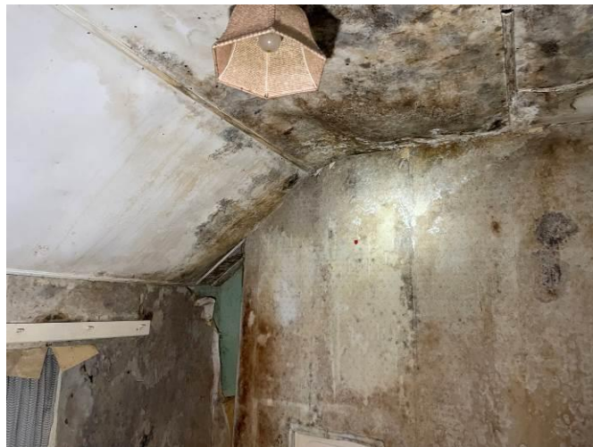
Photograph 25: Typical condition of the internal walls and ceilings within the residential properties
