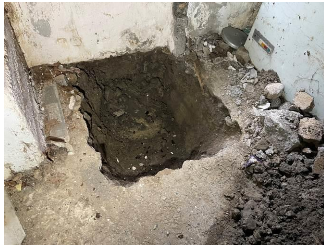
Photograph 7: Shallow depth of bearing stones under external walls of the Basement Area. Formation at 600mm below FFL
