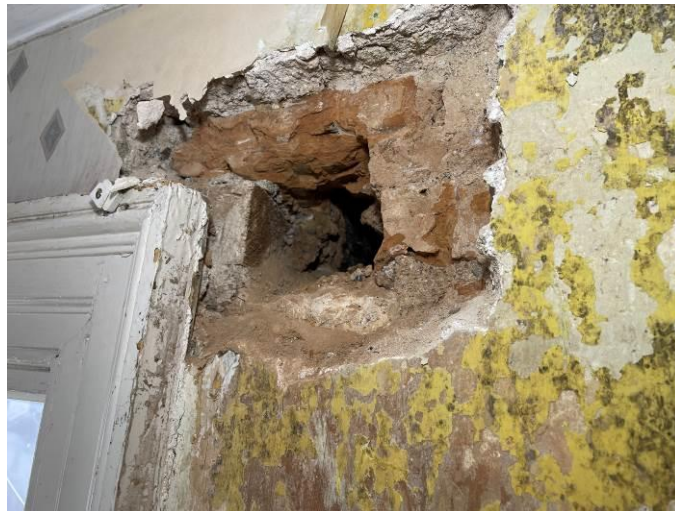
Photograph 17: Typical example of the nature and condition of the timber lintels in the public house area, 1 st floor
