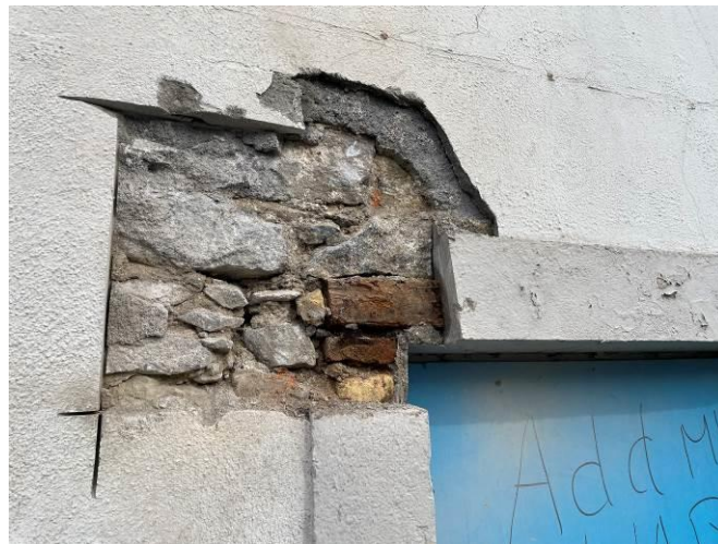
Photograph 20: Note the water damaged timber lintel on the front elevation
