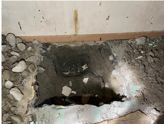
Photograph 6: Shallow depth of bearing stones under external / party walls of residential property adjacent to the Public House. Formation at 600mm below FFL
