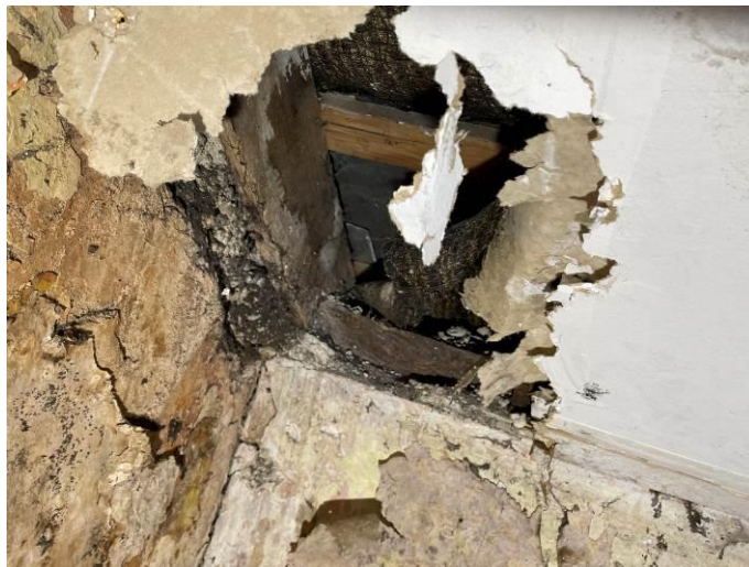
Photograph 46: Dilapidated and water damaged timber rafters in the residential property adjacent to the public house, left side
