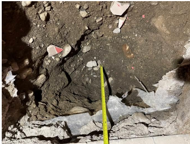
Photograph 4: Shallow depth of bearing stones under external / party walls of the existing dwellings (Unit 01). Typically, formation level is at 700mm below existing FFL
