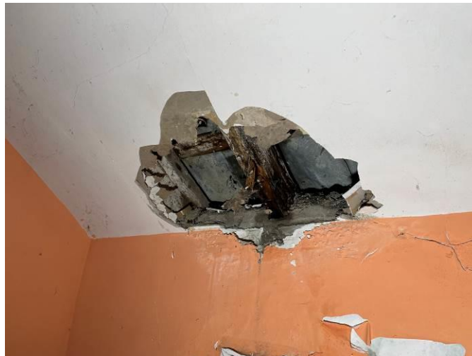
Photograph 41: Example of water damaged ends of rafters in the residential properties and where same abut the external walls
