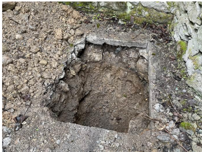
Photograph 2: Typical external ground conditions with good ground encountered at 1m to 1.5m below existing ground level. Note the shallow depth of the bearing pad stones under the stone wall
