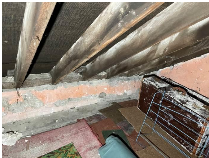
Photograph 44: Good condition of the attic space and timbers in the property adjacent to the public house
