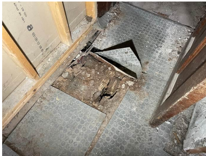
Photograph 36: Close up of the defects noted above
