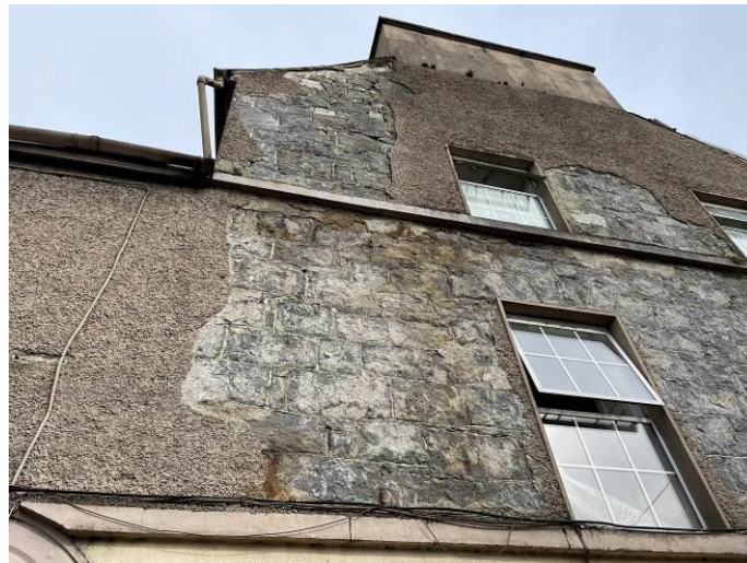
Photograph 23: Spalled render from public house section
