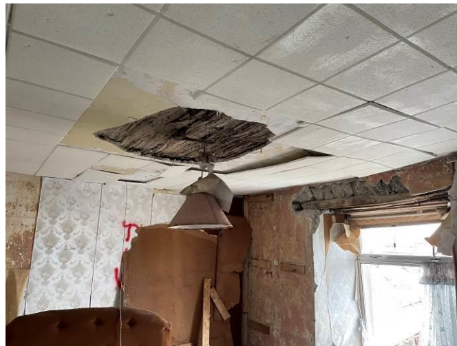
Photograph 27: Dilapidated nature of the walls and ceilings within the public house area
