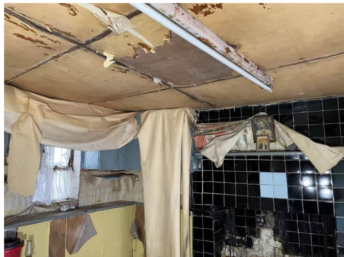
Photograph 28: Dilapidated nature of the walls and ceilings within the public house area
