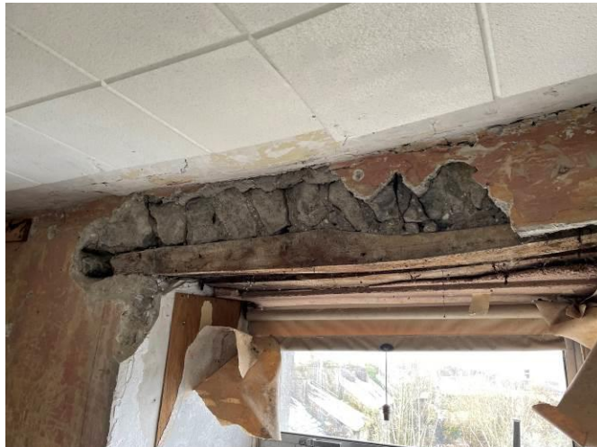
Photograph 14: Woodworm noted in timber lintels within the public house part of the property
