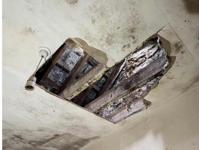
Photograph 40: Dilapidated condition of the roof and attic spaces in the residential properties
