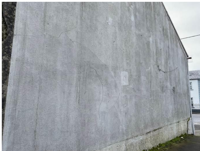
Photograph 18: Cracked and hollow sounding render noted on the left side gable end of the residential properties
