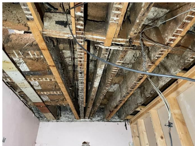
Photograph 37: Condition of the timber first floor joists in the public house area
