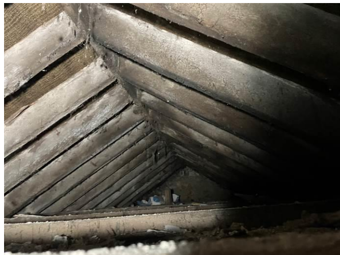
Photograph 47: Good condition of the rafters in the roof over the public house area
