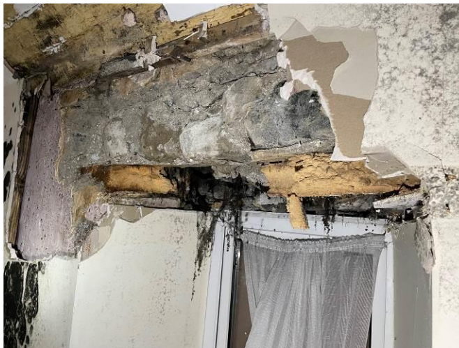
Photograph 11: Example of rotted and dilapidated timber lintel
