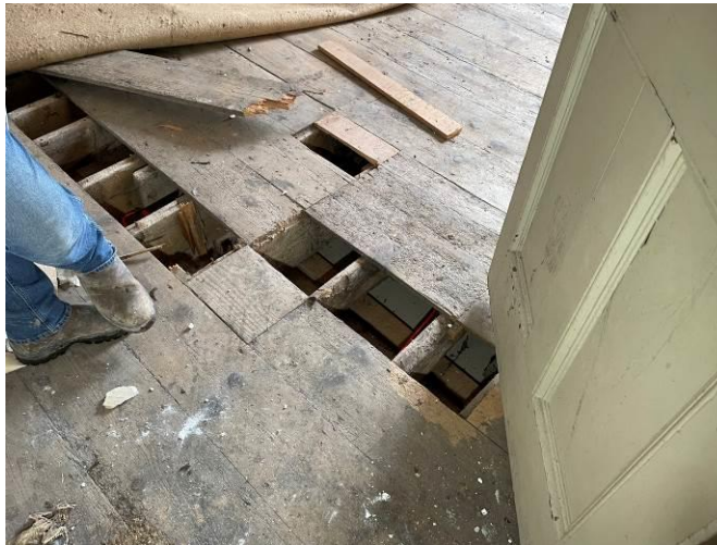
Photograph 33: Brittle condition of the floorboards and floor joists in the property adjacent to the archway
