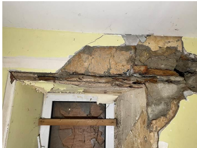
Photograph 9: Condition of Timber Lintels in Unit 03
