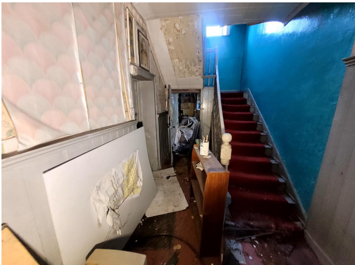
Figure 3. Shows the ground floor of the Three Storey Townhouse. Note the base of the stairs is in poor condition.
