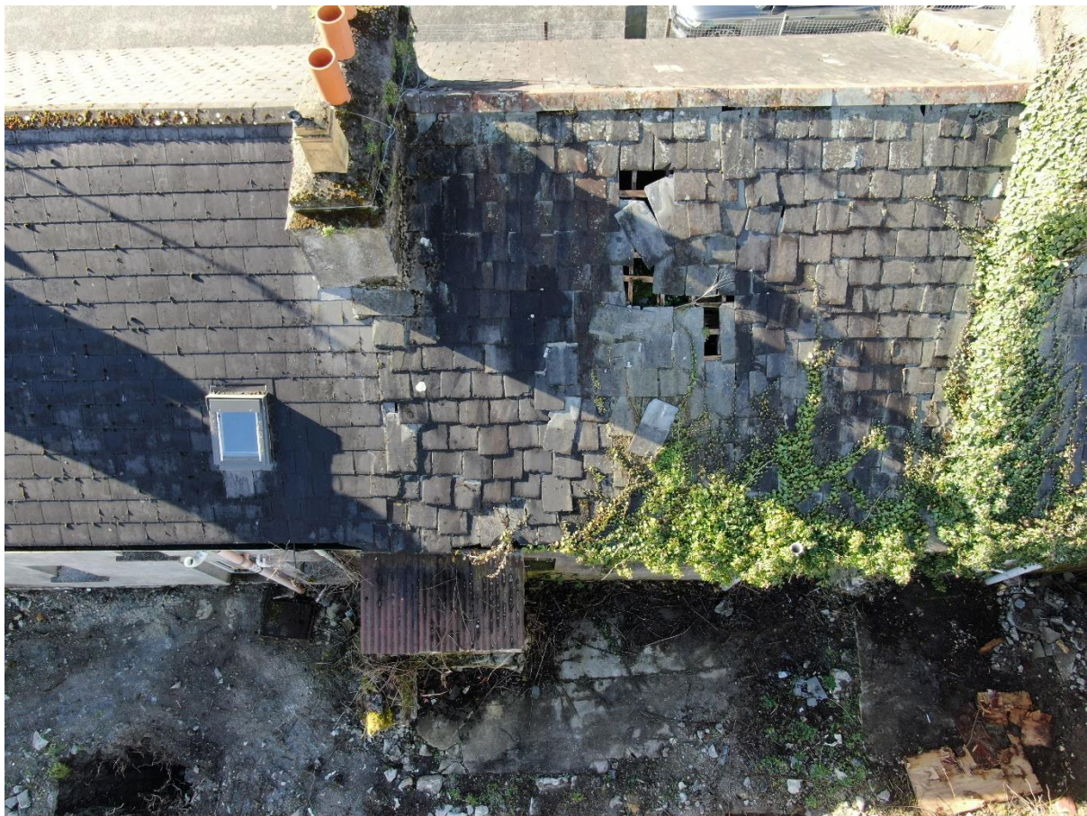
Figure 18. Shows an aerial view over a typical cottage that is in poor condition.
