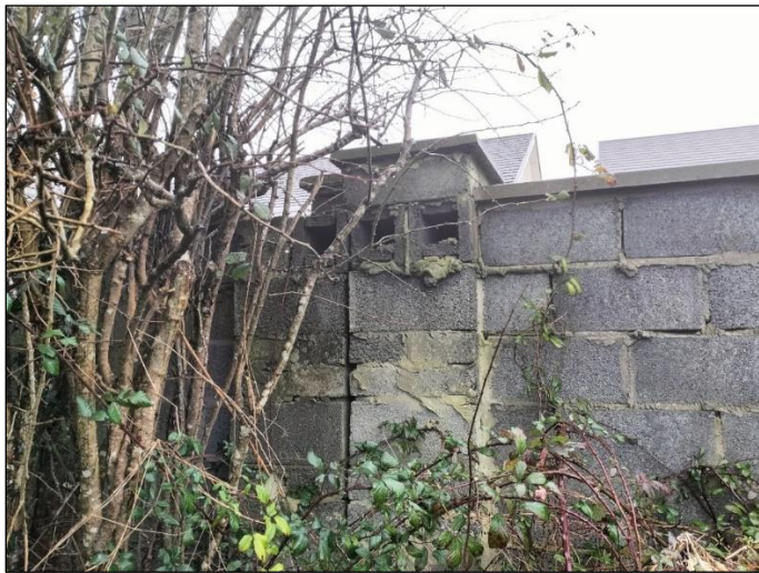
Plate 5-12 Concrete block wall located to the north of the development site with some visible gaps.
