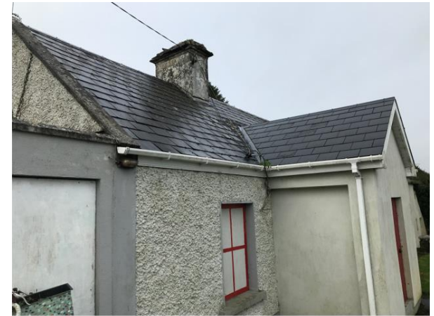
Plate 3: View of slate roof in good condition with no obvious access points to the interior
