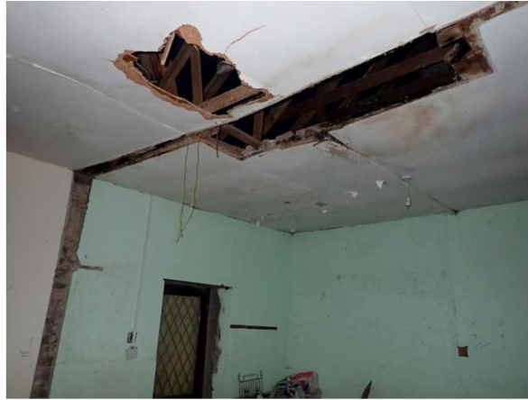
Plate 8: View of degraded ceiling during March 2024 survey
