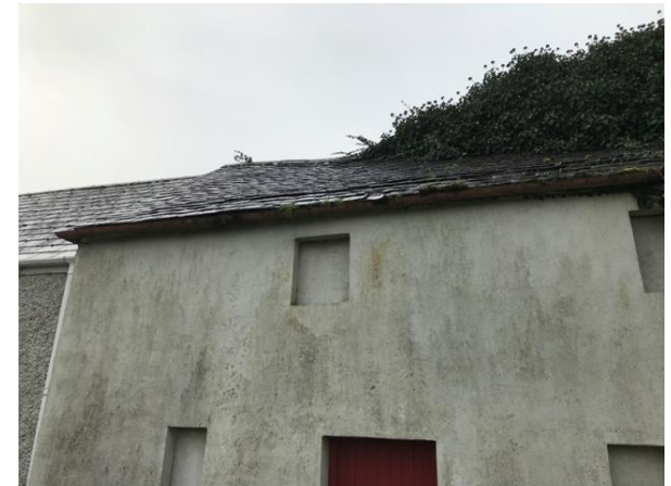
Plate 6: View of adjoining shed area with uneven slates but no obvious access points on the front elevation.
