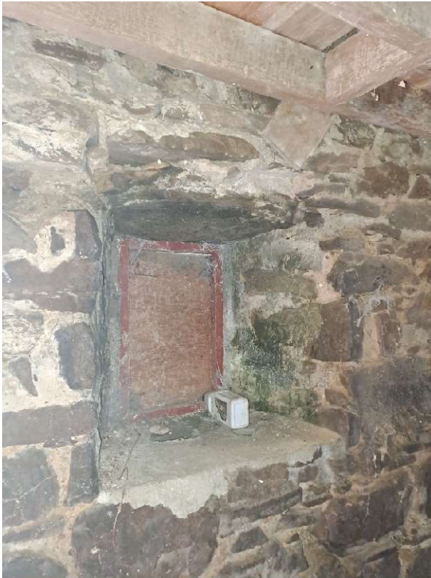
Figure 5- Structural supports missing to internal head of window ope 1
