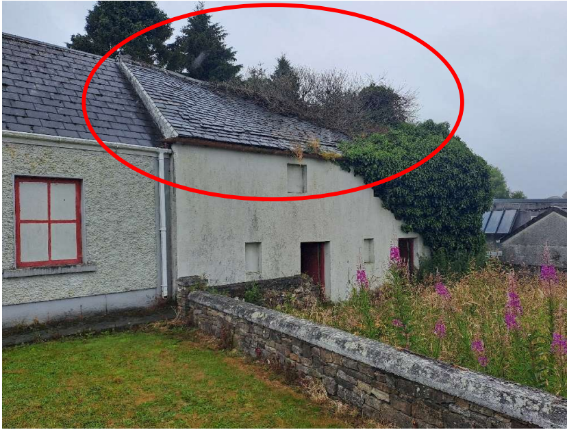
Figure 13- Significant Ivy growth with visible undulations in the roof structure
