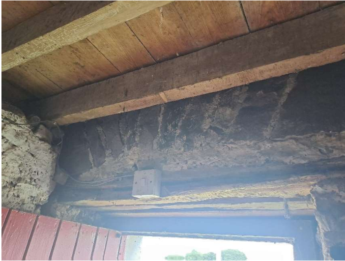
Figure 7- Evidence of intervention to original arched door opening head
