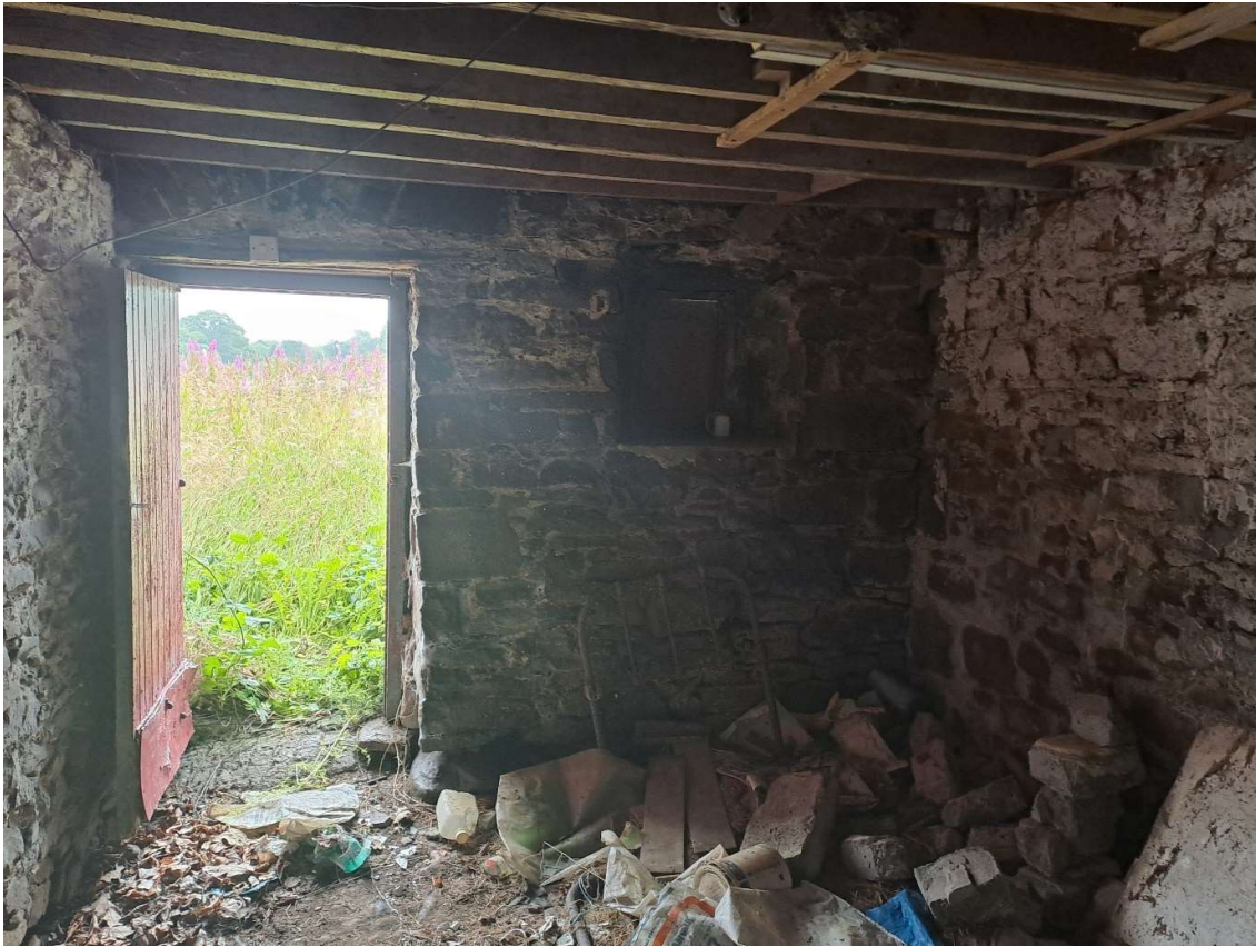
Figure 3- Overview of stone structure missing adjacent to door ope threshold
