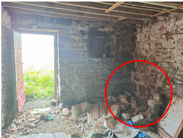
Figure 10- Significant mortar infill to base of wall
