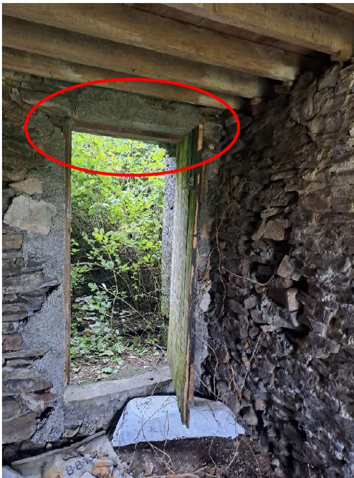
Figure 19- Evidence of intervention to original rear wall to create a door ope (no structural lintel to head)
