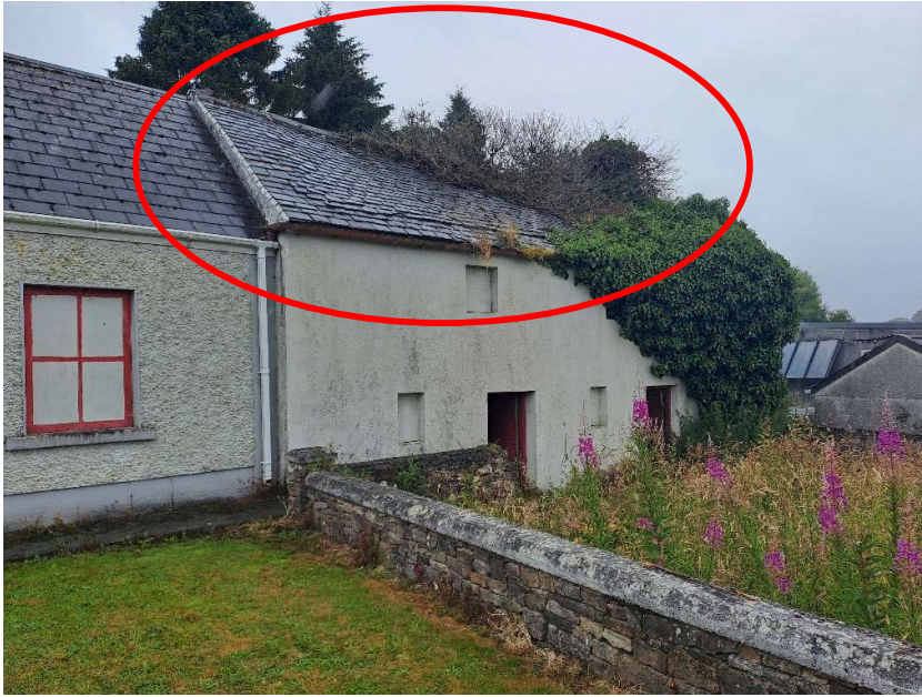
Figure 24- Significant Ivy growth with visible undulations in the roof structure
