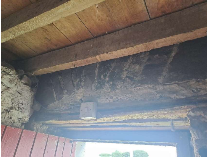
Figure 18- Evidence of intervention to original arched door ope head
