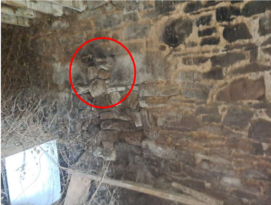
Figure 22- Missing Keystone to original fireplace ope
