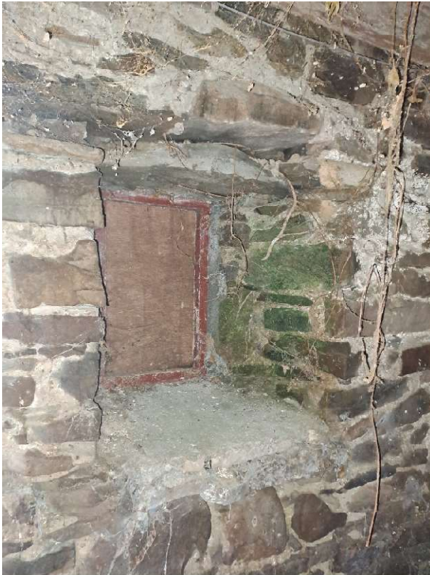
Figure 6 - Structural supports missing to internal head of window ope 2
