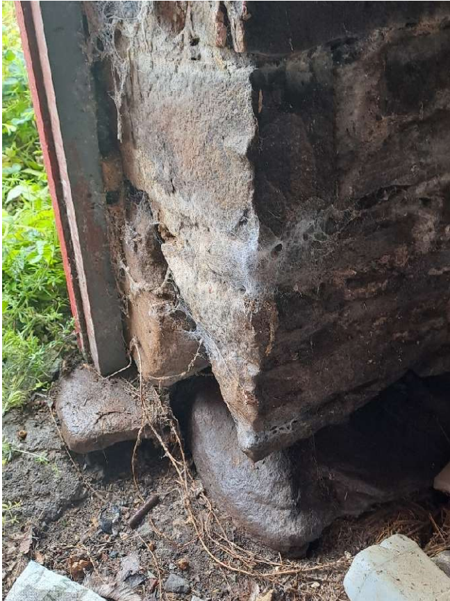
Figure 15- Detail view of stone structure missing adjacent to door ope threshold
