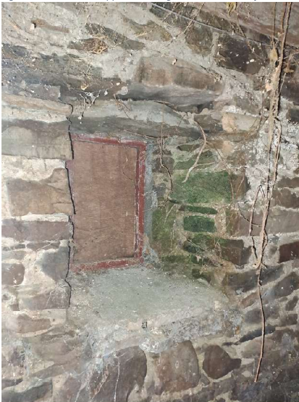
Figure 17 - Structural supports missing to internal head of window ope 2
