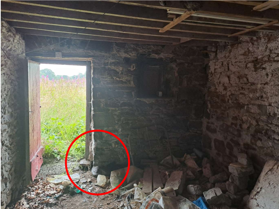
Figure 14- Overview of stone structure missing adjacent to door ope threshold
