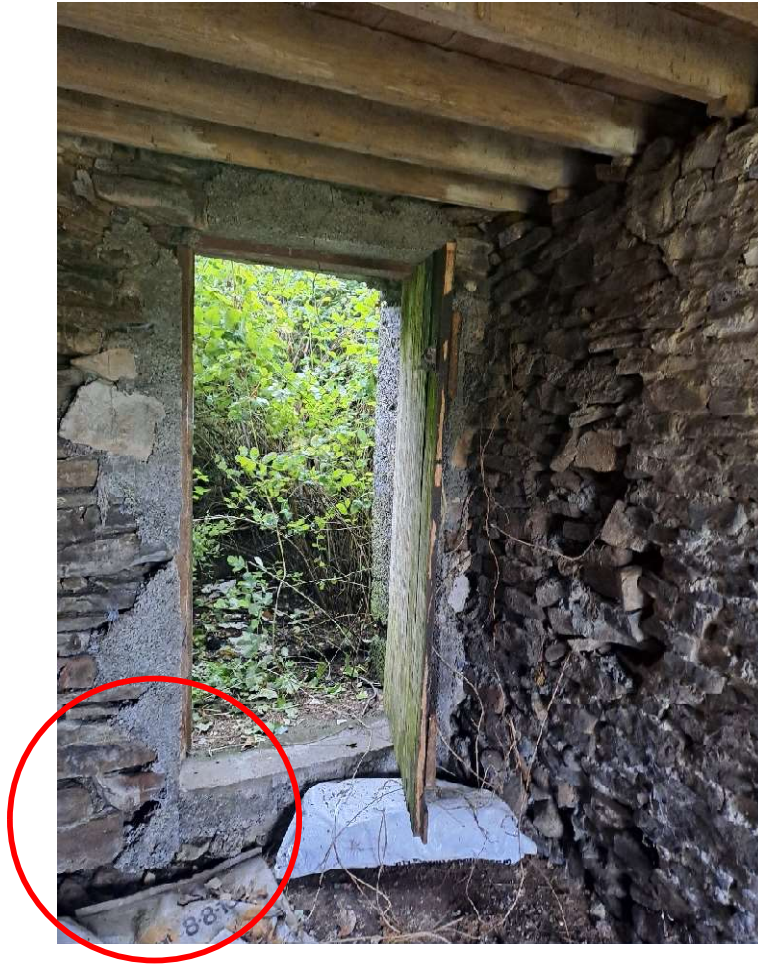
Figure 9- Smaller stones at foundation level than that of the supported wall
