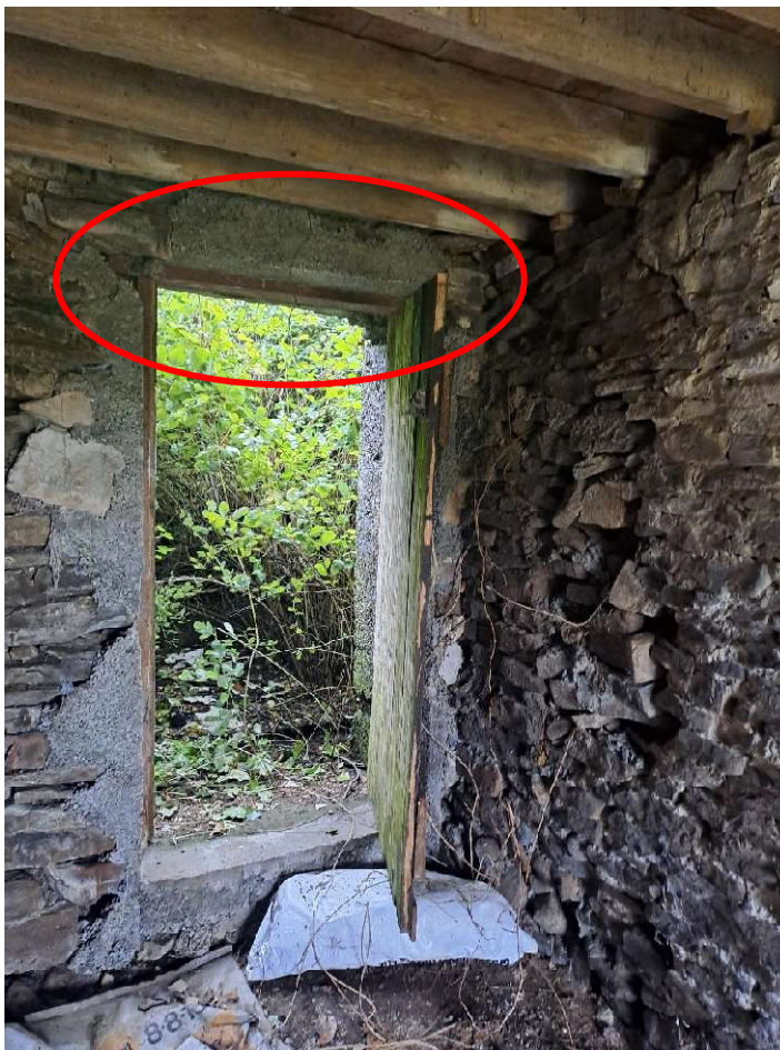
Figure 8- Evidence of intervention to original rear wall to create a door opening (no structural lintel to head)
