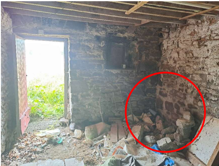
Figure 21- Significant mortar infill to base of wall
