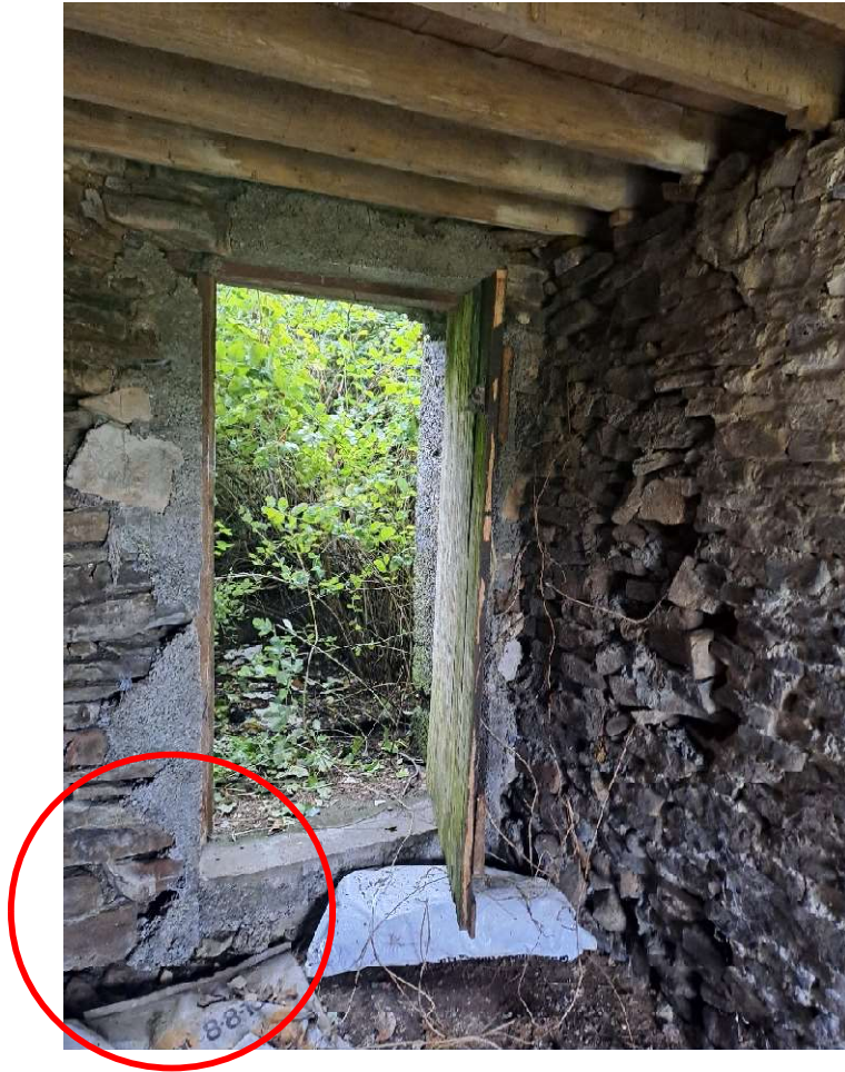
Figure 20- Smaller stones at foundation level than that of the supported wall
