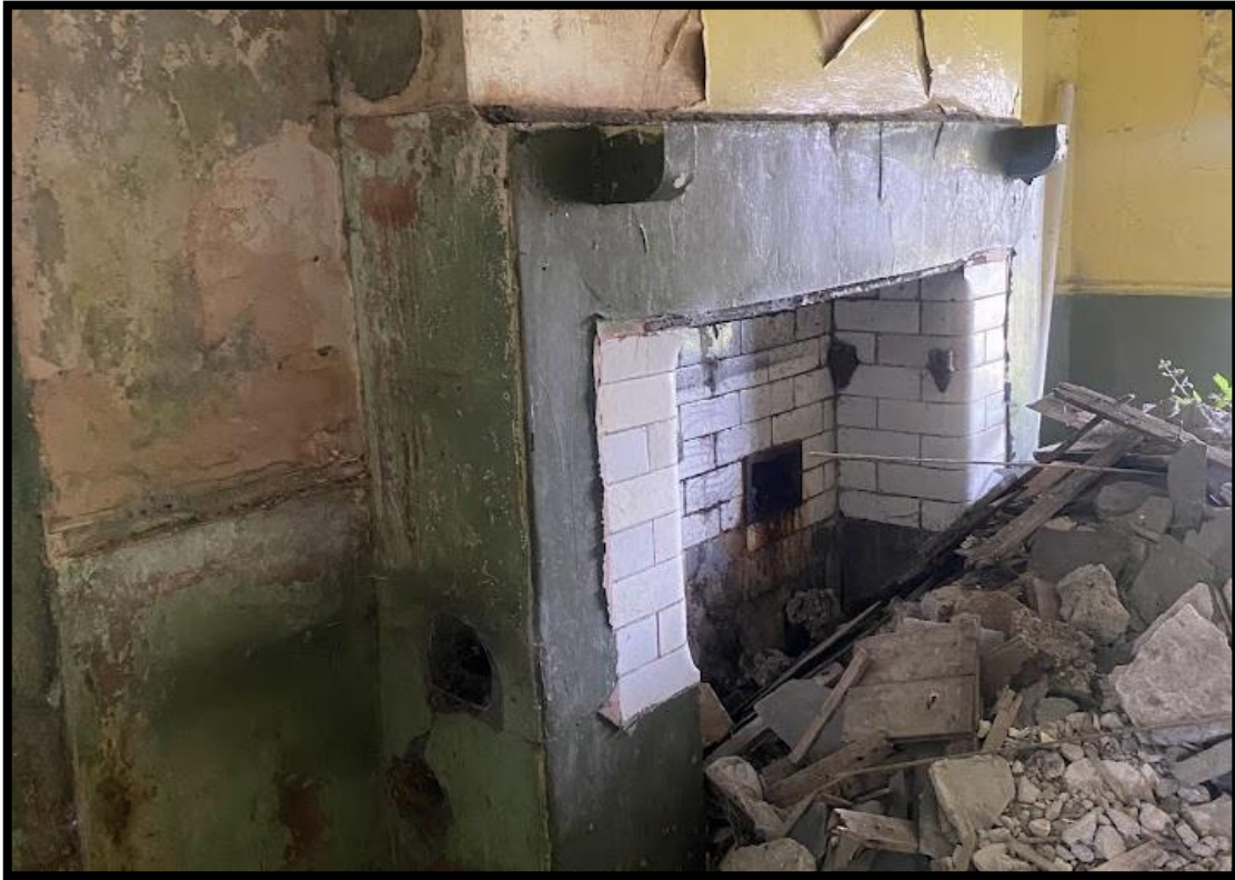
Figure 6.8- Chimney and rubble to the rear of building 2
