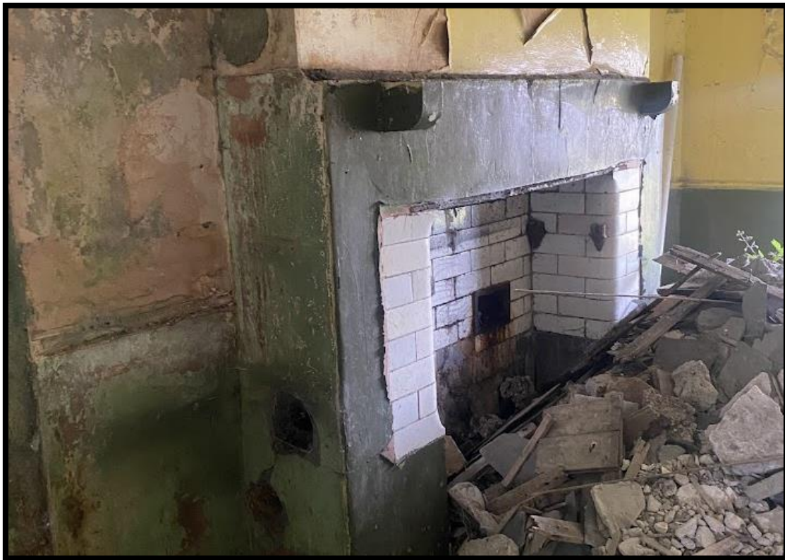
Figure 2.10- Chimney and rubble to the rear of building 2
