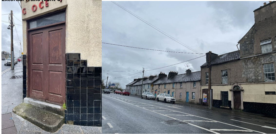
OBFA photos of existing ceramic tiled wall finish to external ground level walls of Dooley's Pub
