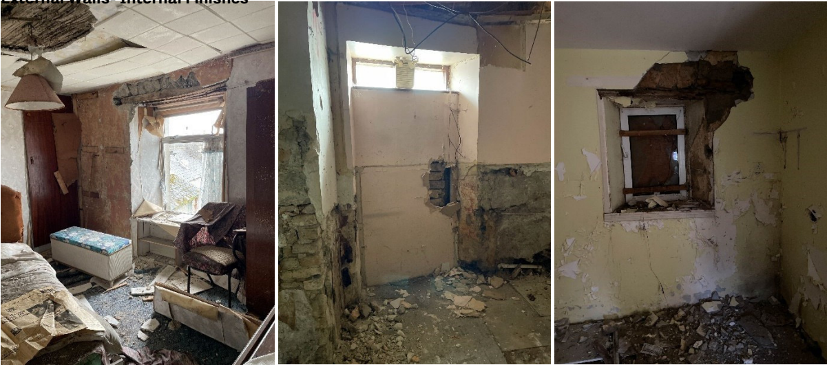
OBFA photos of inner faces of typical existing external walls
