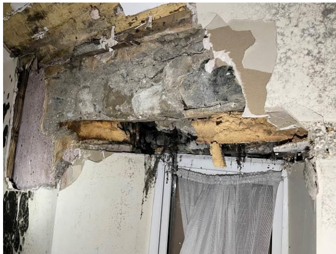
Photograph 11: Example of rotted and dilapidated timber lintel
