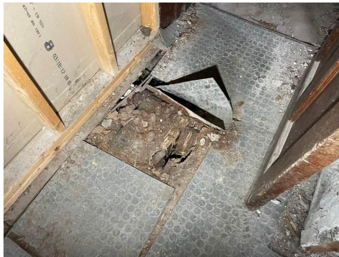
Photograph 36: Close up of the defects noted above
