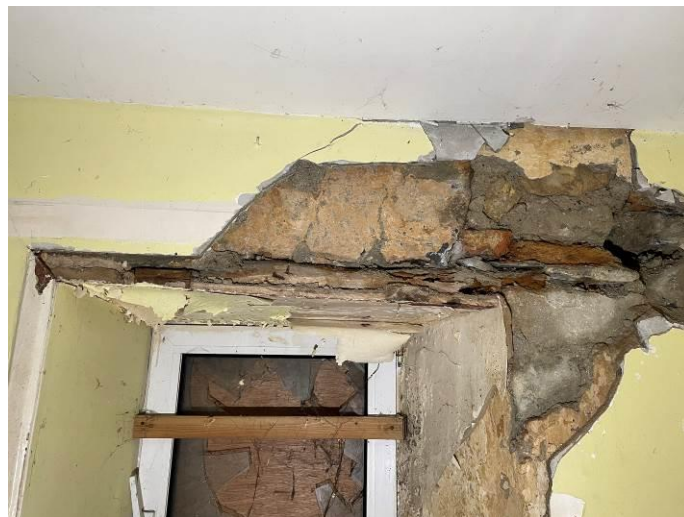
Photograph 9: Condition of Timber Lintels in Unit 03
