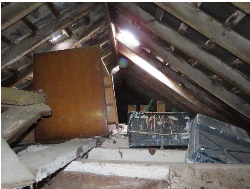
Photo 33 - Attic of Property 4 with void in roof
