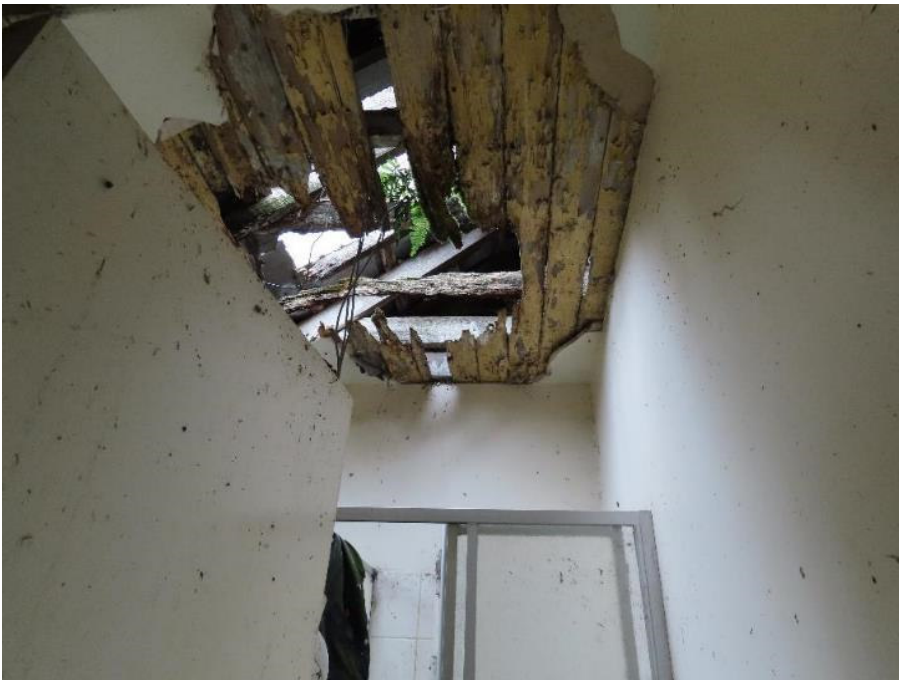
Photo 38 – damage to ceiling in Property 6
