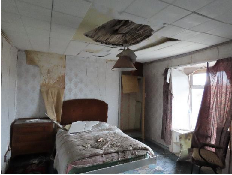
Photo 57 – bedroom with damaged ceiling
