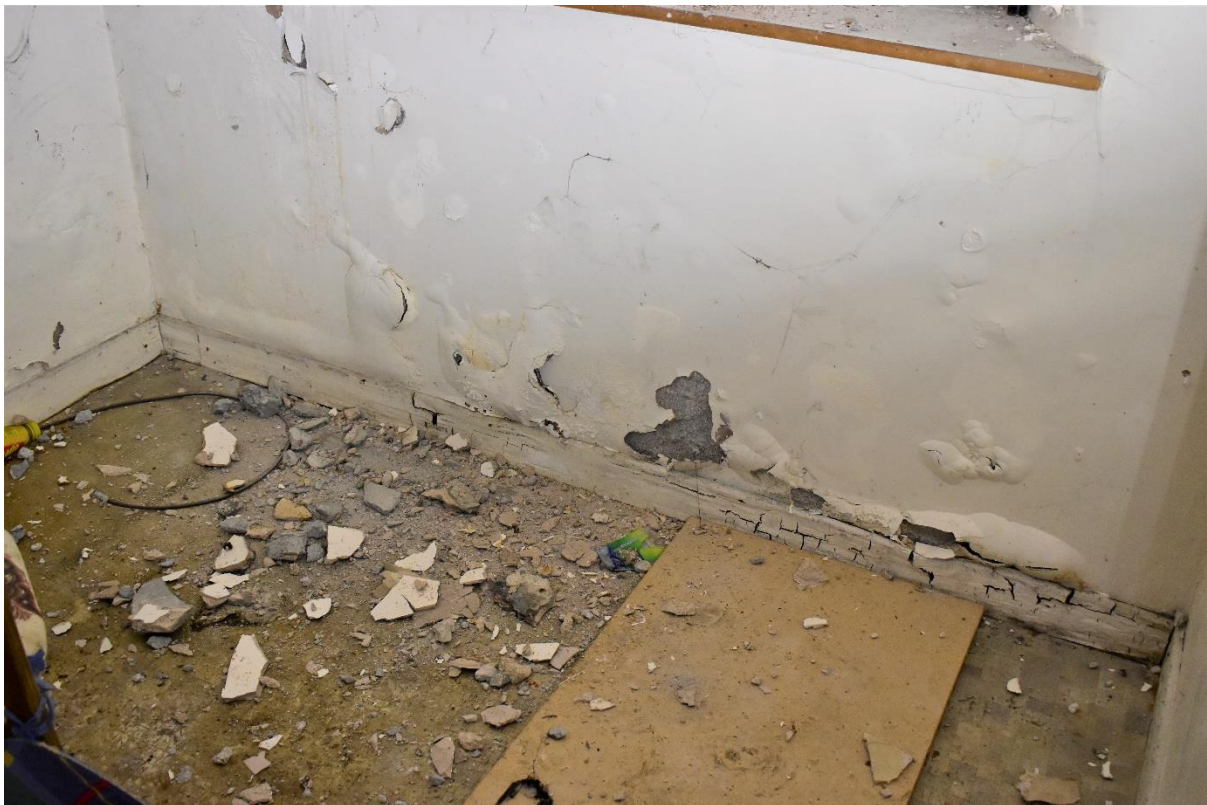
Figure 19. Shows a typical section at the base of the masonry in a cottage from rising dampness.
