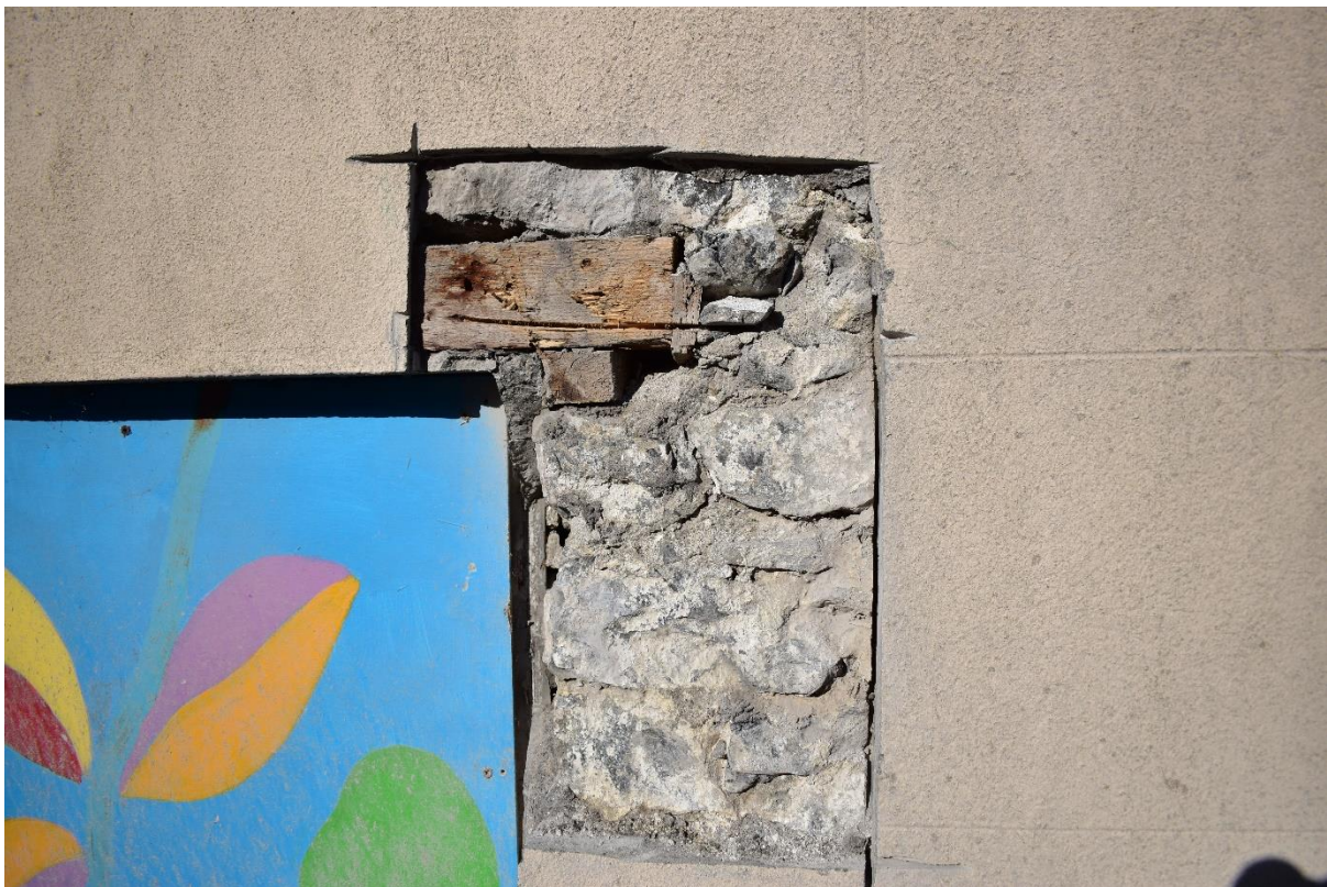
Figure 20. Shows a section of removed render that has exposed an external timber.
