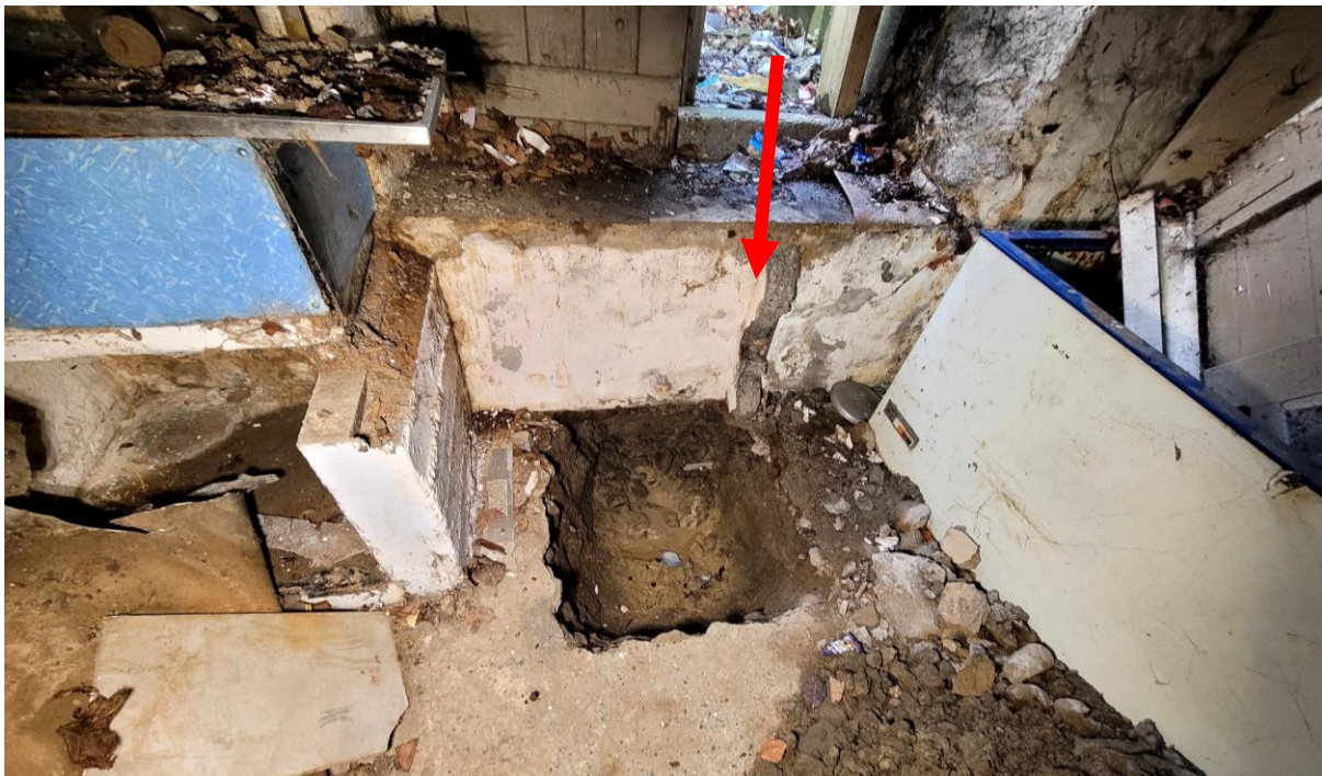
Figure 8. Shows the area exposed in the basement. Note the water ingress through the light well.
