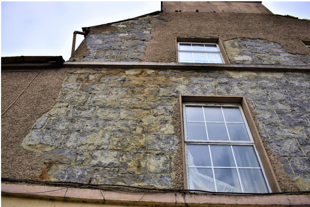
Figure 17. Shows the external of Dooley's Pub where the render has blown. Note the staining from the chimneys.
