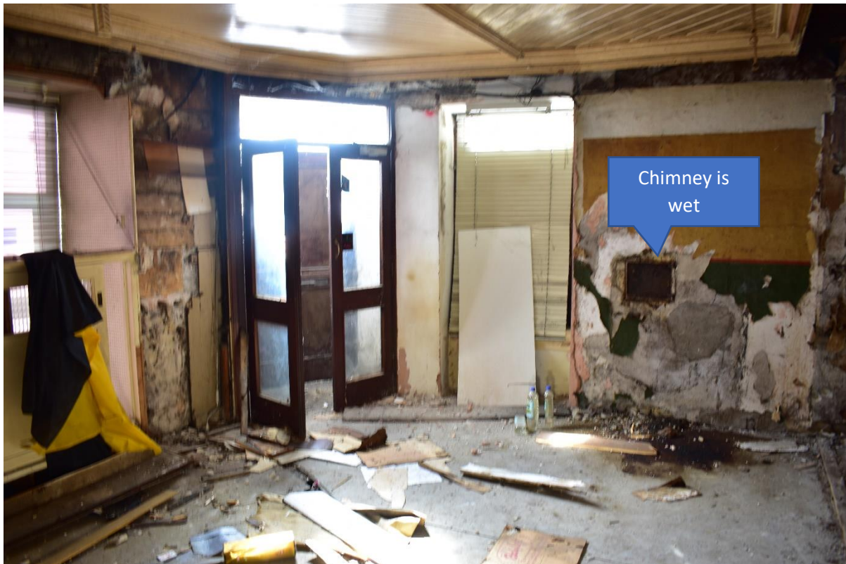
Figure 11. Shows a broad view of the ground floor, including a section of the chimney that is currently wet.
