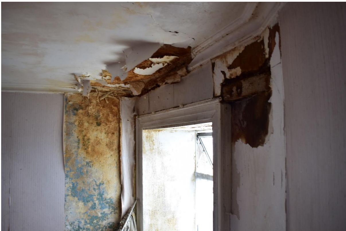
Figure 21. Shows a section of deterioration from salts bleeding through from the chimney at the second floor level in Dooley's Pub.
