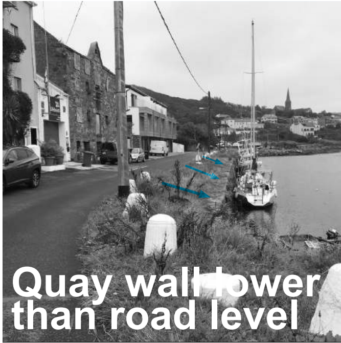
The Quay wall appears to be considerably lower than the level of the road. This will need to be managed carefully to ensure the quay is accessible and safe.
