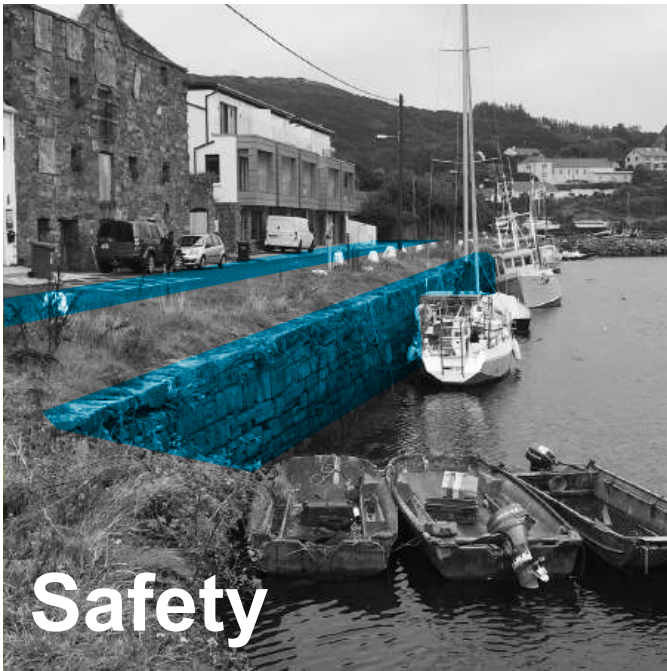
The Quay wall and Beach Road pose potential safety risks to pedestrians.
