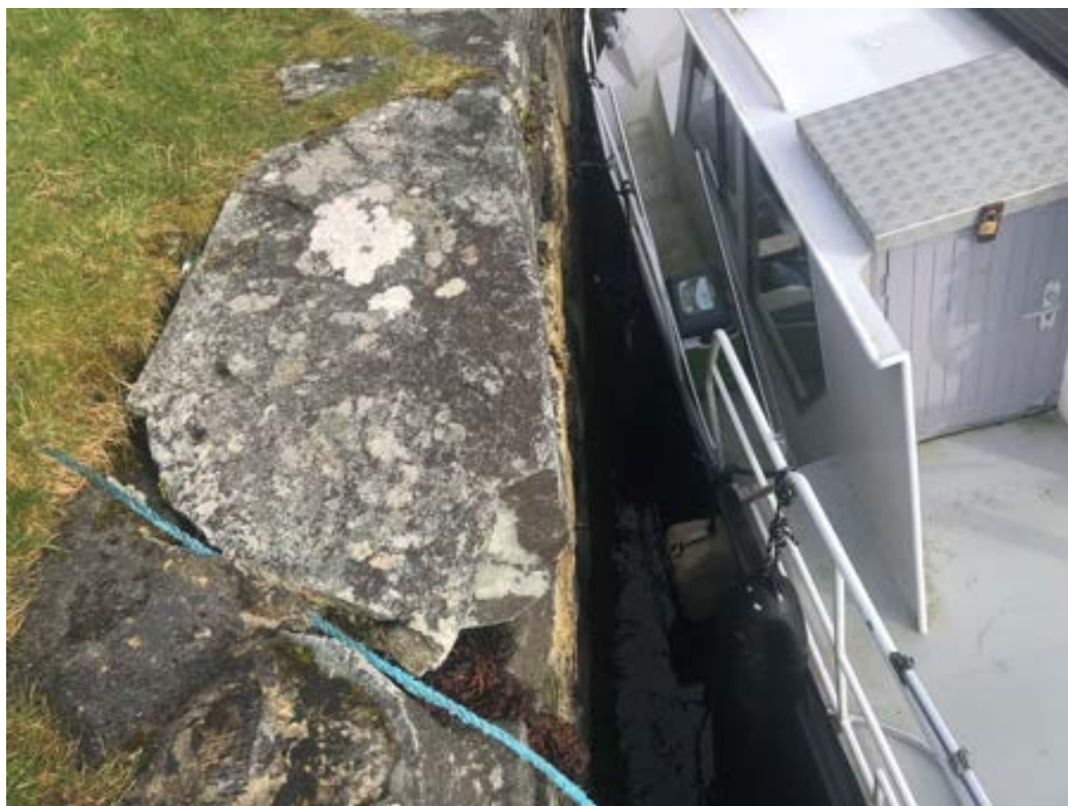
Figure 2 - Capping stones dislodge by mooring lines
