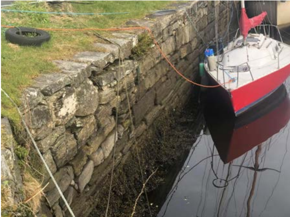
Figure 3 - Vegetation and stonework dislodged
