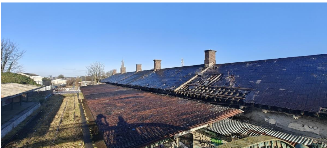
Plate 3-2: Rear view of buildings roof including multiple holes providing potential access
