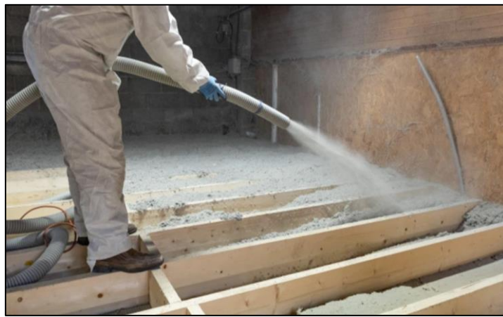
Photograph 12: Example of Cellulose being sprayed in between ceiling joists in an attic 3
