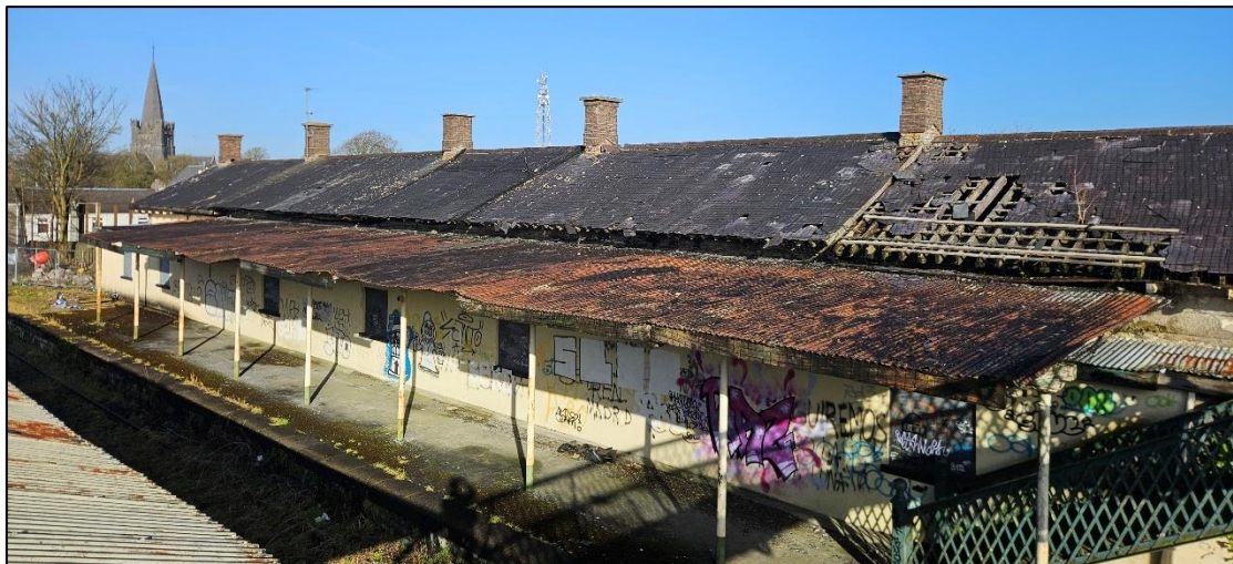
Photograph 2: View of the western roof planes in very poor condition
