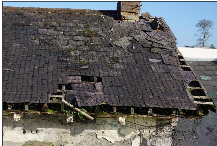
Photograph 3: View of decayed roof timbers
