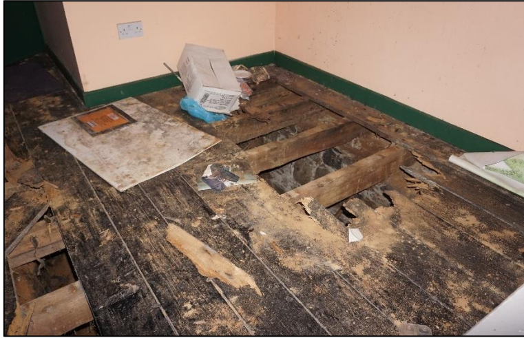
Photograph 6: View of a suspended timber floor in very poor condition
