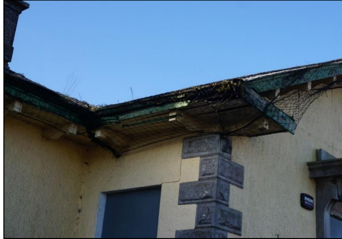
Photograph 5: View of blocked and rusted cast iron gutter
