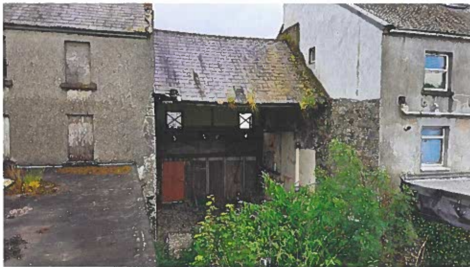
Photograph 7 Roof of Building "A". Rear elevation, only supported by the party walls.
