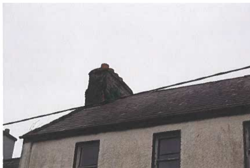
Photograph 5 Chimney Stack on party wall between Buildings “A” and “B”. Natural Stone Construction exposed under the failed render.
