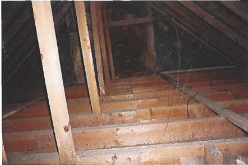
Photograph 14 View of chimney system within the roof space. Note migration of soot to the external face of the chimney liner masonry.
