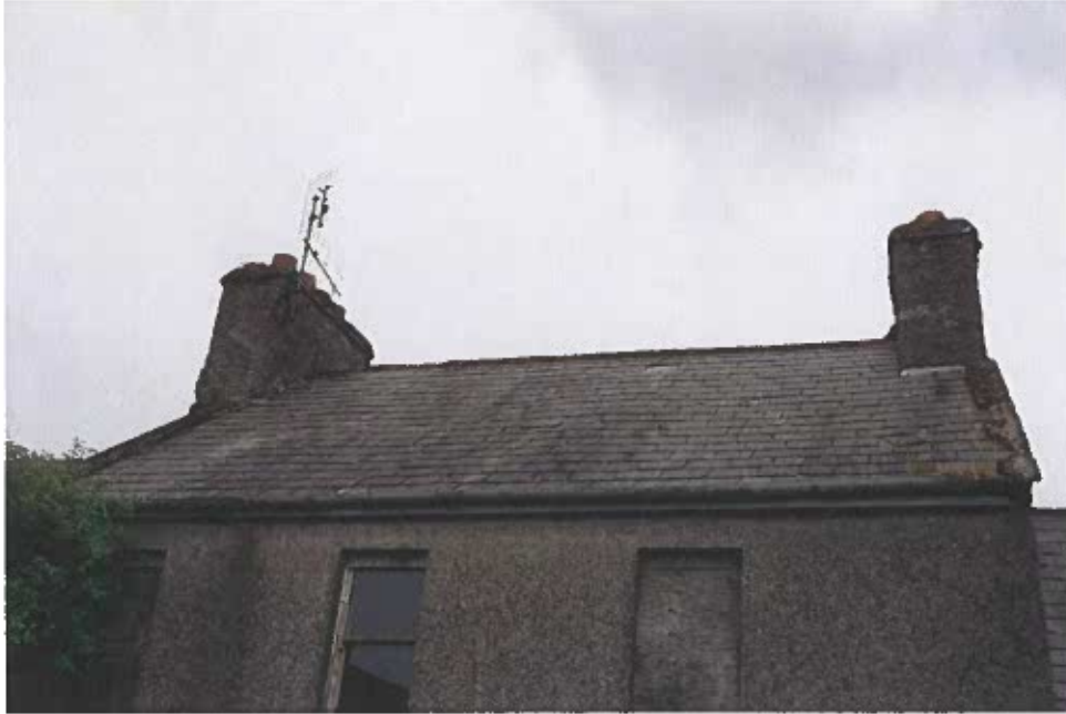
Photograph 17 Rear roof plane of building “B”. Natural slate covering. Note condition of concrete barges.
