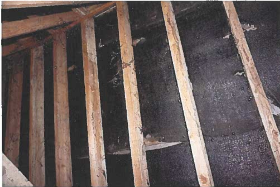
Photograph 16 View of the underside of the roof covering. Bituminous felt in very poor repair, natural slate covering on view.
