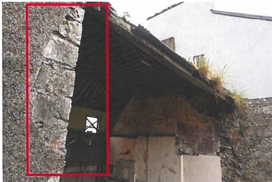
Photograph 20 View into building "A". Note exposed masonry beneath the failed render of building "B".
