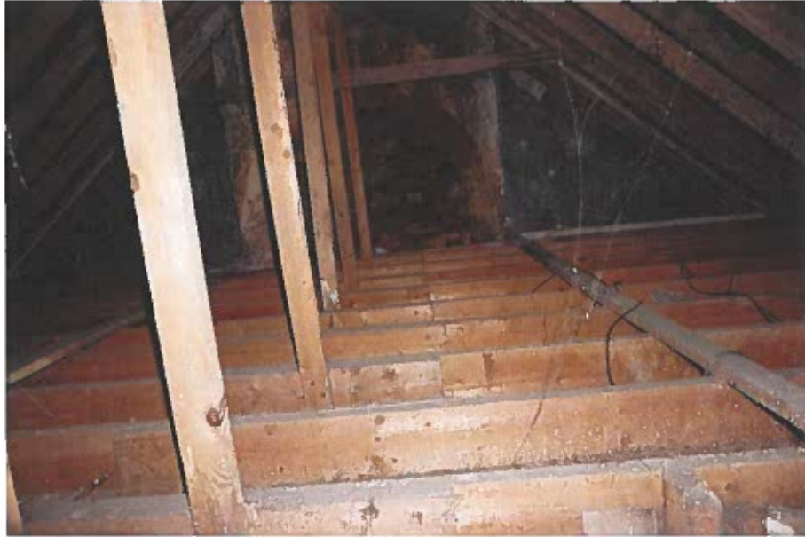
Photograph 6 Chimney system of Buildings "A" and "B". Note staining.
