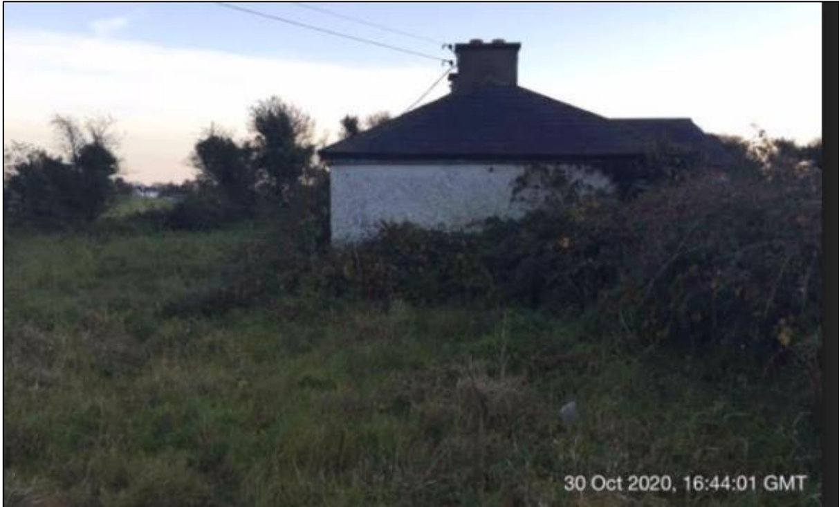
Photograph 2: Flank Elevation of The Existing Dwelling taken from within the site boundary
