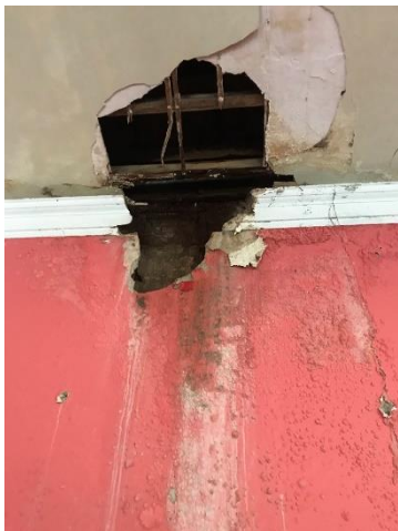
Photo 46. Ceiling and wall damage
