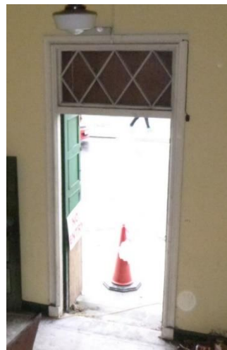
Photo 11 & 12. Ground Floor Cinema windows & Main building entrance doors lattice fan light window
