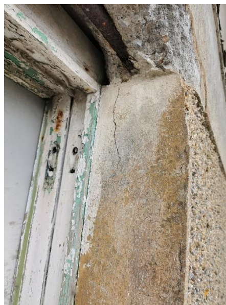
Photo 13 & 14. First Floor Level Ballroom windows with steel bar as protective barrier. Spalling concrete lintol
