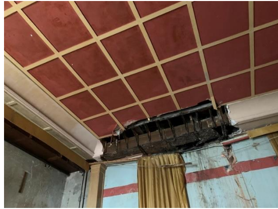
Photo 36. Cinema ceiling and water damage
