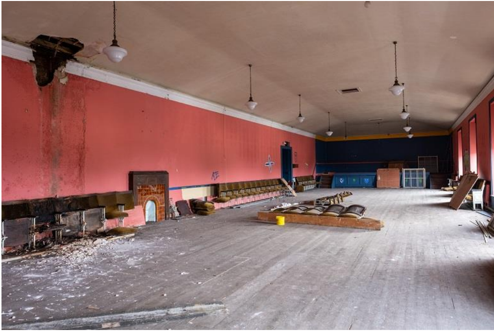
Photo 25. The Ballroom interior looking east (note water damage at ceiling)
