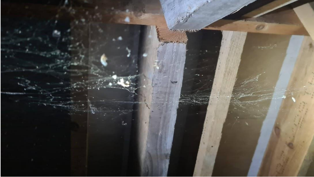
Plate 3-5 Accumulation of cobwebs in attic space
