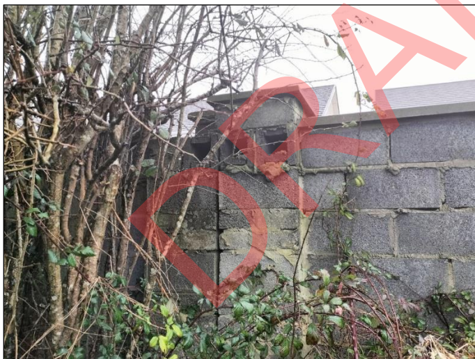
Plate 5-12 Concrete block wall located to the north of the development site with some visible gaps.
