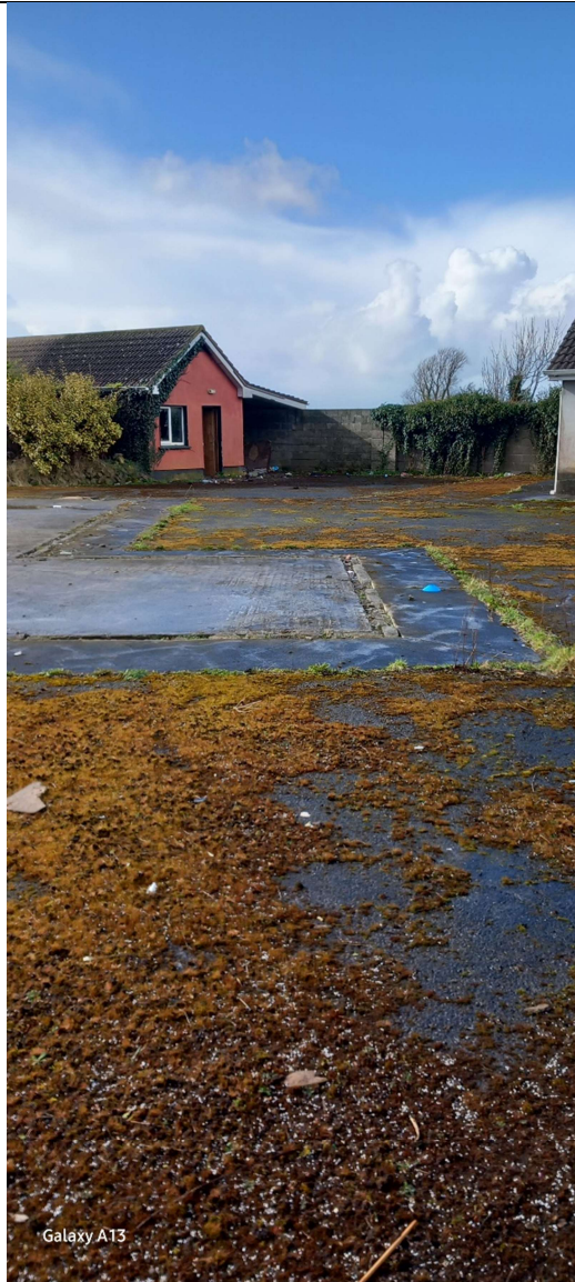
Figure 3.4 - Existing Shed ( Lean to roof to be demolished to comply with planning)
