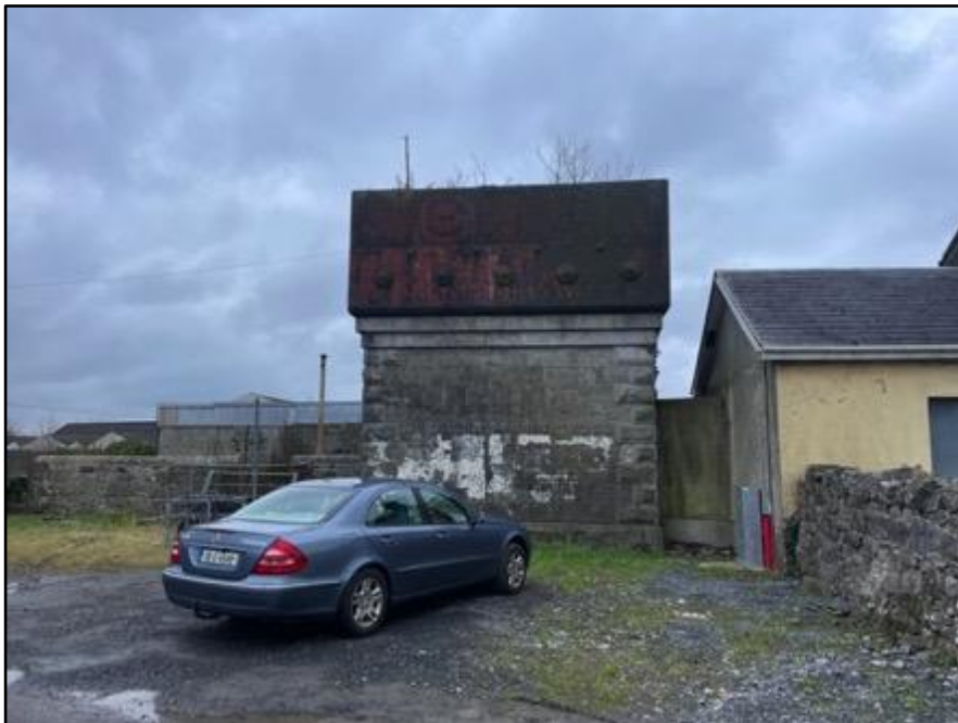
Plate 4: Tank located to the immediate SE of the station building. Taken from the E.
